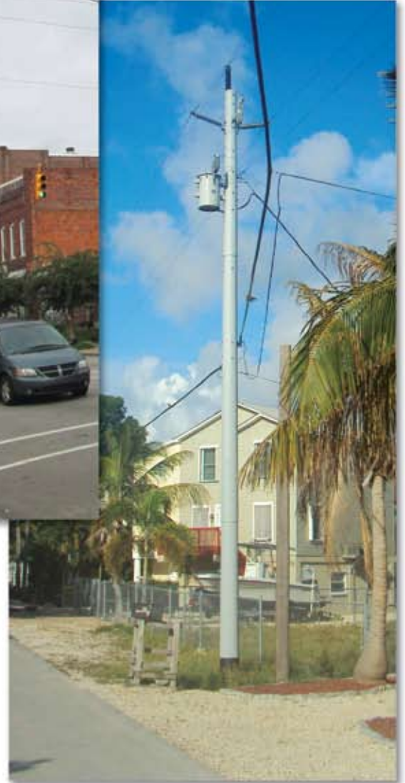
Corrosive Environments & Coastal Areas
