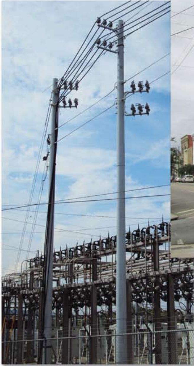
Transition out of Substations
